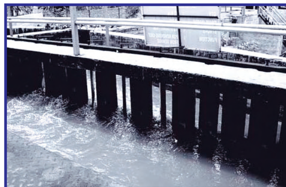
Fig.13.4 Grit and sand removal tank
