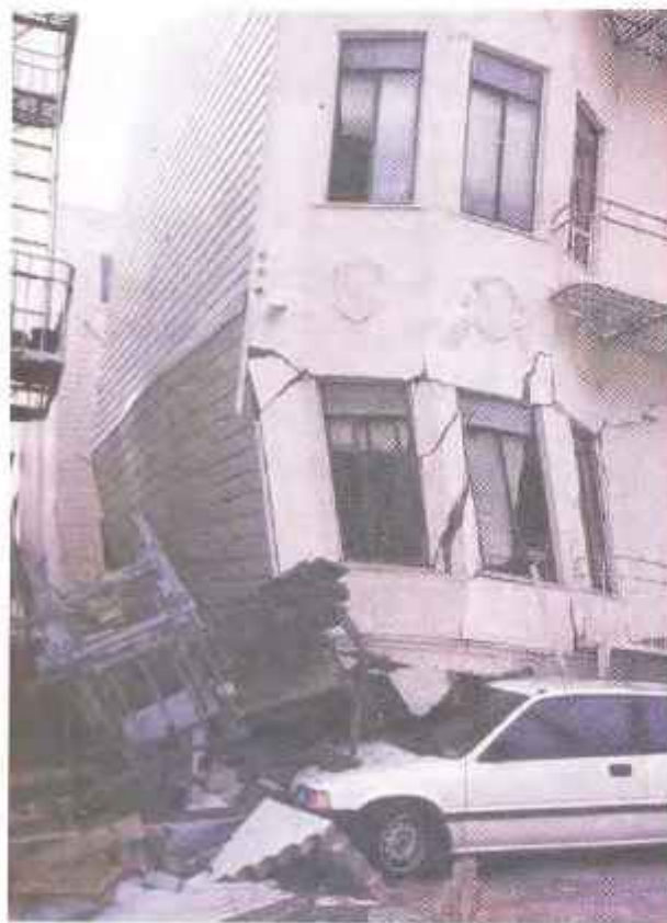
An earthquake can damage buildings
